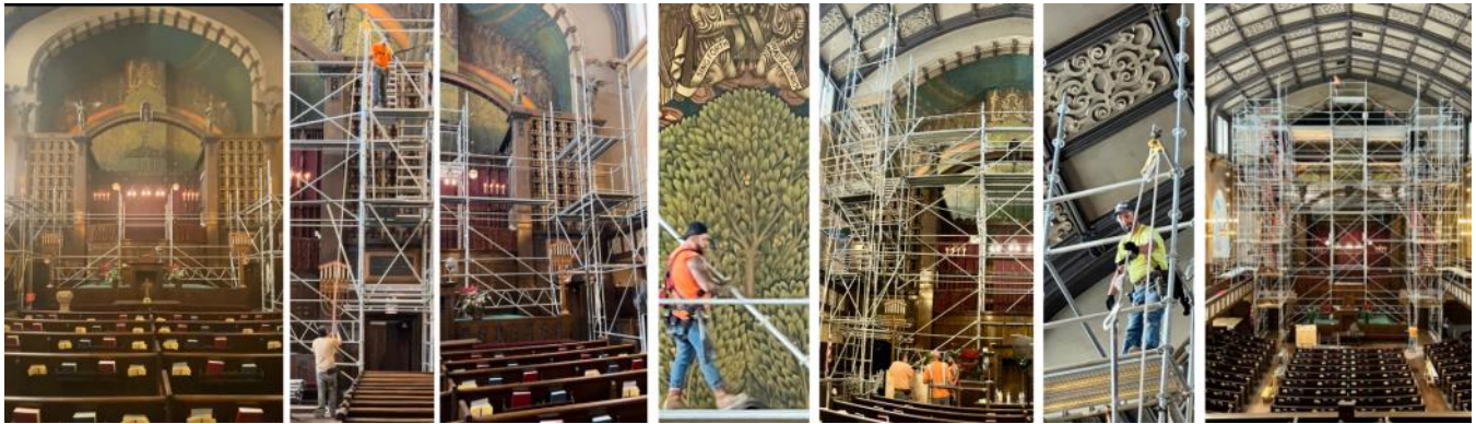
This set of photos shows the transformation timeline of the build out of the scaffolding. The first photo far left is day one of the build out. The second photo left shows Gilco Scaffolding Company using a pulley system to deliver materials. The third photo is half way finished. The fourth center photo shows Angel an employee of Gilco carrying pipe. Finally, the fifth photo is of the build-out which is three quarters of the way finished, the sixth photo shows the top of the pulley system with a bar being lifted, and the seventh photo far right is the total build out of the scaffolding.
