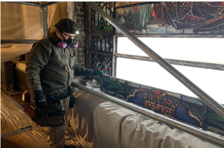
Jim Murphy removing the first pieces of Tiffany's original 1895 St. Paul Stained glass window.
